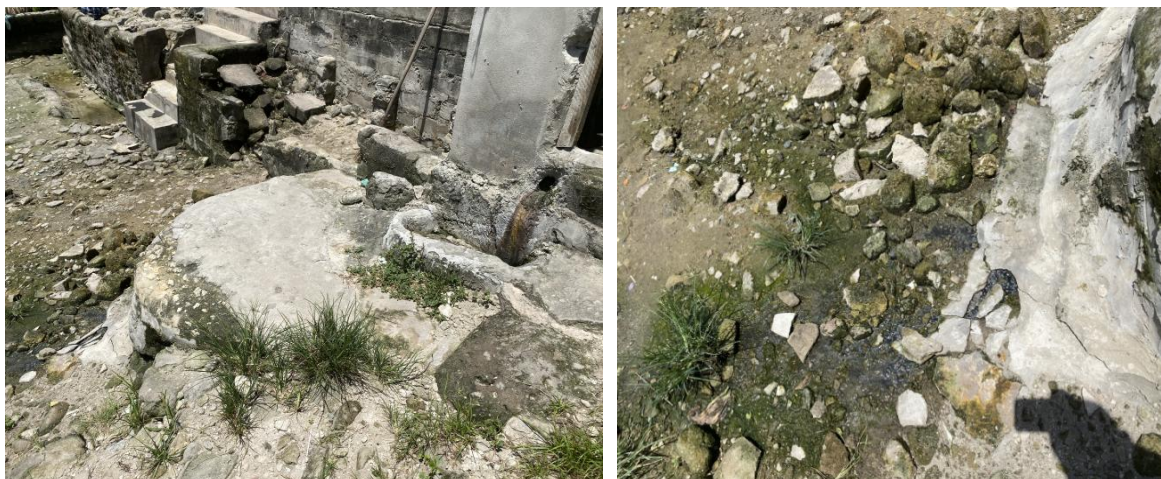
Fig. 3. Leakage in a sanitation facility
